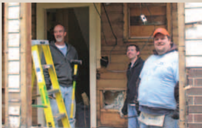
Volunteers from Sunnyside Mennonite work on the front porch of a house on S. 12 th Street.
